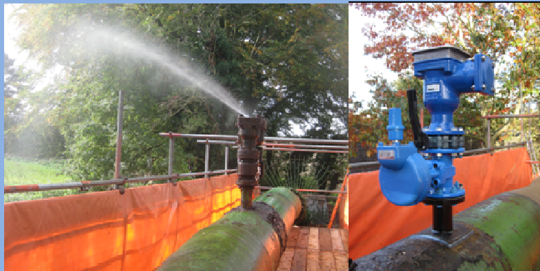
Example of air valve pre and post intervention
